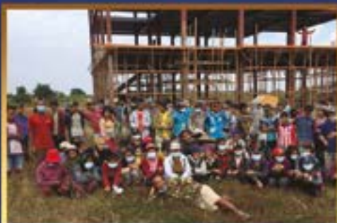
We have maintained our construction schedule during COVID and the Civil Disobedience Movement. Most of these workers would have no income if we were to stop building. This has given us great influence into the construction workers' world, as we represent Christ to them.
