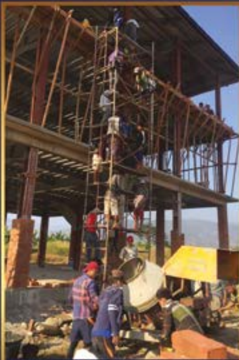
There were 183 workers on site to help pour the third floor. They worked into the early morning hours to complete the job.
