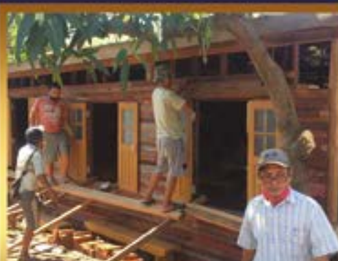
Men work on another expansion of our Harvest Church Kalaymyio. We have had to expand the building four times to meet the church's growth.
